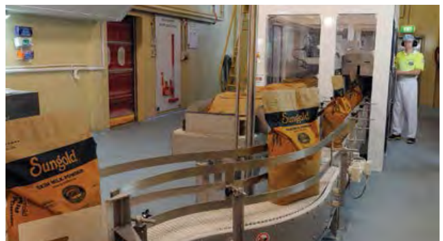
This year a new powder packing line – the first of its kind in Australia – was installed in WCB's powder plant.
