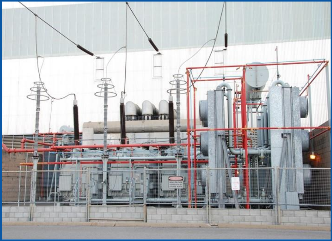
Typical Power Station Generator Transformer
