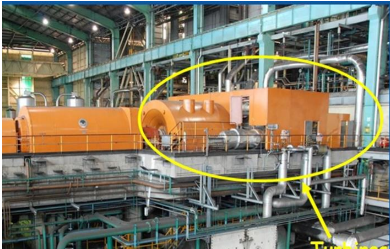
Typical Power Station Turbines
