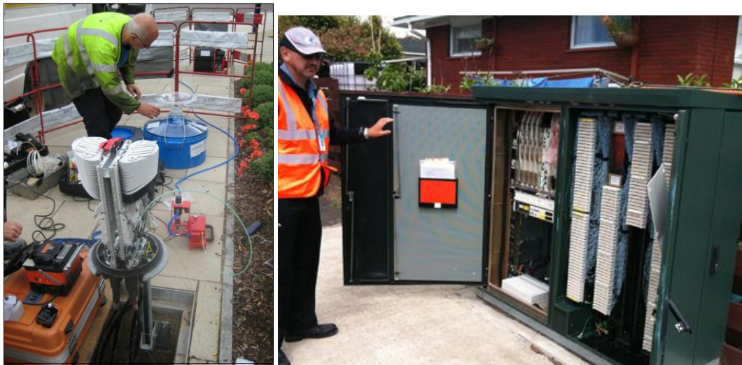
Figure 3.5: Underground enclosure (left) and street cabinet (right) for splitters [Source: Analysys Mason]
