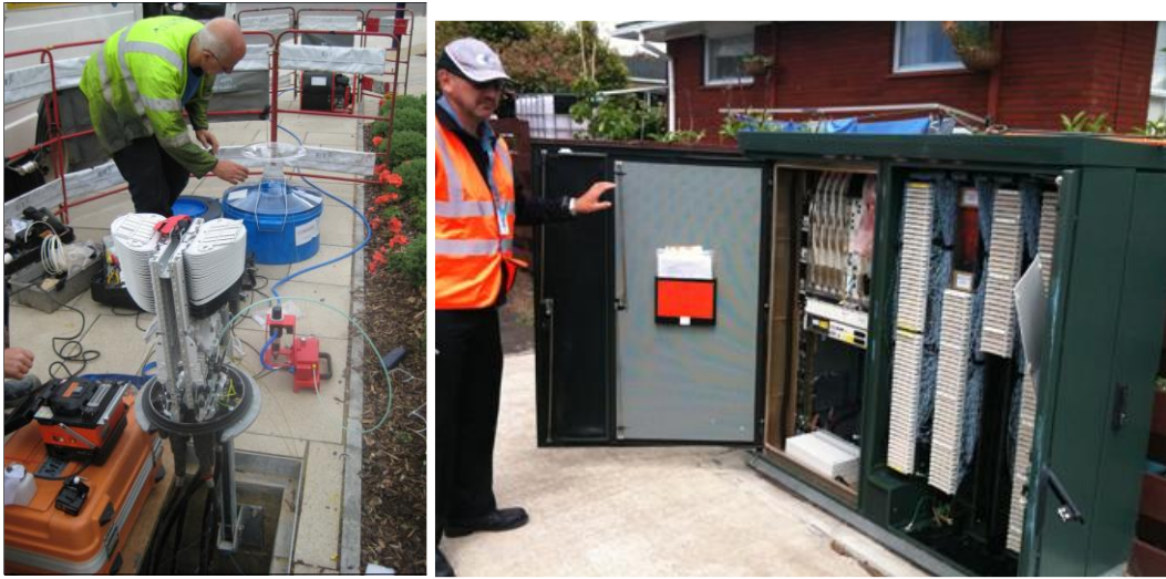
Figure 4.5: Underground enclosure (left) and street cabinet (right) for splitters [Source: Analysys Mason]
