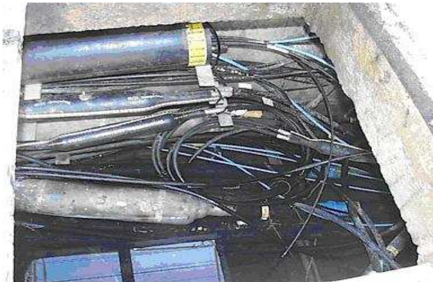
MANHOLE NEAR CNR FERNTREE GULLY RD & LUM RD, WHEELERS HILL (27-SEP-2001) NOTE OPTICAL FIBRE JOINT ENCLOSURE (TOP) AND COPPER CABLE JOINT ENCLOSURES (LOWER) AS WELL AS NUMEROUS SMALLER SIZE CABLES (REFLECTION OF SKY IN WATER AT BOTTOM)
