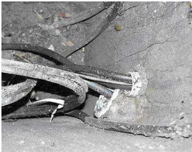
PLASTIC PIT AT CNR AJAX DR & BELINDA CR, WHEELERS HILL (27-SEP-2001) CLOSE UP VIEW OF CONDUIT EXITS AT RIGHT WITH MULTIPLE CABLES NOTE CABLE TV COAXIAL CABLE RUNNING VERTICALLY IN LOWER RIGHT CORNER
