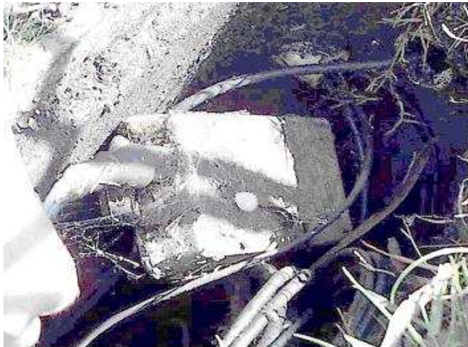
PIT OUTSIDE 23 BELINDA CRES, WHEELERS HILL (27-SEP-2001) CUSTOMER LEAD-IN PIPE AT LEFT, STREET PIPE AT TOP SMALL PAIR GAIN SYSTEM INSIDE RECTANGULAR CASE
