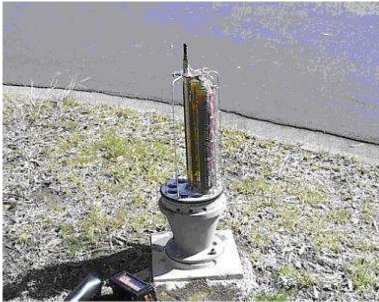
'900' TYPE PILLAR (P85) CNR AJAX DR & DONALD ST WHEELERS HILL (27-SEP-2001) NOTE CABLE TERMINATION STRIPS AND SPARE PORTS (HOLES) FOR ADDITIONAL STRIPS (100 PAIRS / STRIP)
