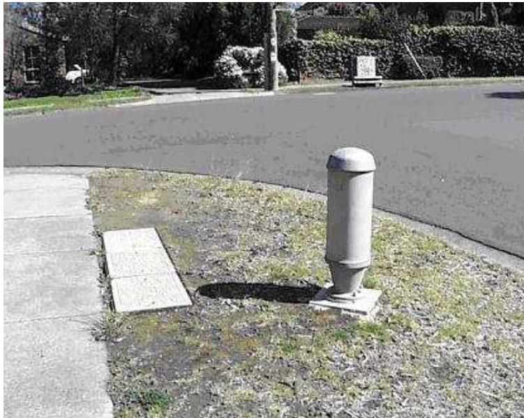
'900' TYPE PILLAR AND '9' PIT CNR AJAX DR & DONALD ST WHEELERS HILL (27-SEP-2001)
