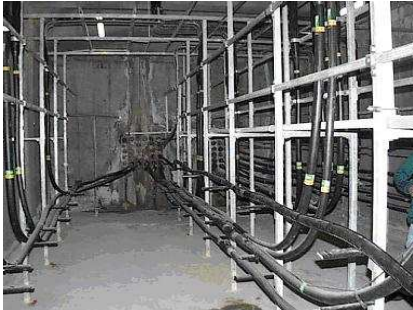
MORDIALLOC EXCHANGE CABLE CHAMBER (16-SEP-1999) NOTE MAIN CONDUIT ENTRY AT END OF CHAMBER AND LARGE QUANTITIES OF LARGE COPPER CABLES ENTERING AND PASSING UP UNDERNEATH MDF
