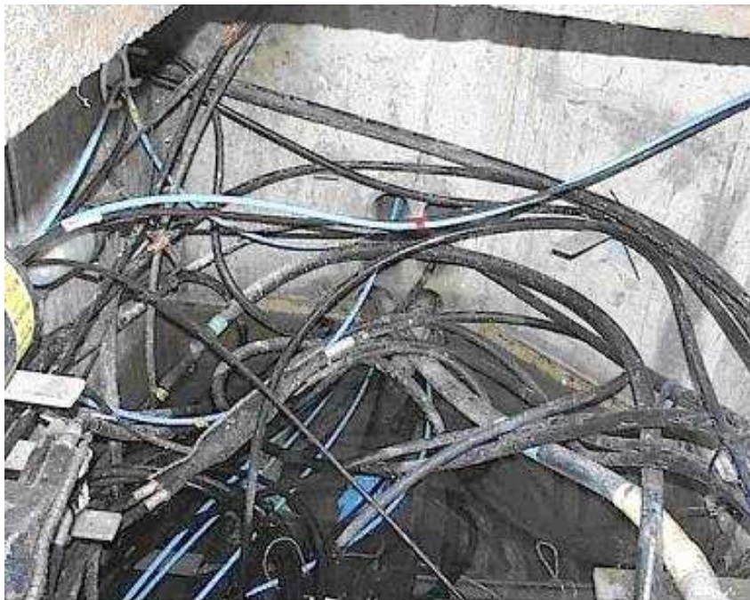
MANHOLE NEAR CNR FERNTREE GULLY RD & LUM RD, WHEELERS HILL (27-SEP-2001) NOTE MAIN CONDUITS AT CENTRE AND LEFT
