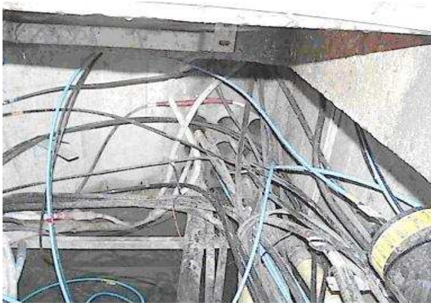
MANHOLE NEAR CNR FERNTREE GULLY RD & LUM RD, WHEELERS HILL (27-SEP-2001) NOTE MULTIPLE MAIN CONDUITS WITH LARGE SIZE COPPER CABLES AND OPTICAL FIBRE (OPTICAL FIBRE JOINT ENCLOSURE IN FOREGROUND)
