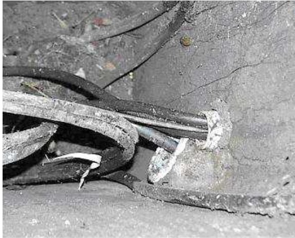
PLASTIC PIT AT CNR AJAX DR & BELINDA CR, WHEELERS HILL (27-SEP-2001) CLOSE UP VIEW OF CONDUIT EXITS AT RIGHT WITH MULTIPLE CABLES
