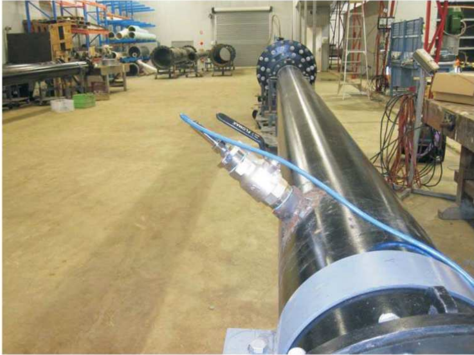
MACE FloPro3 installed in DN300 pipe
