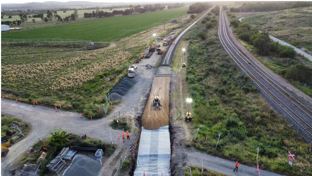
Photo: Bengalla Track Upgrade delivered by external contractors, internal resources & national plant
