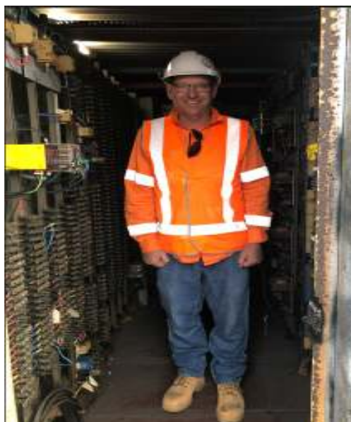
Figure 1: Track worker performing duties in redundant signalling hut with significant safety risk being exposed to live cables within centimetres of his body.
