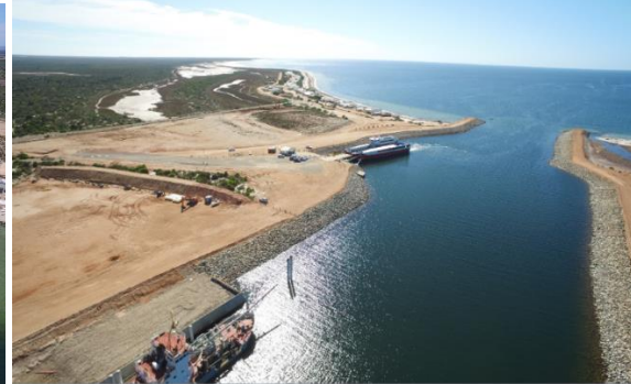
Figure 3: Lucky Bay wharf development – Note: Ferry at berth and dredge at common user export facility berth
