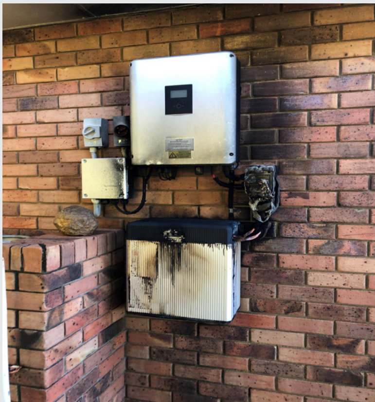
Source: Homeowner affected by the incidents arising from an ESS Home Energy Storage System Battery
