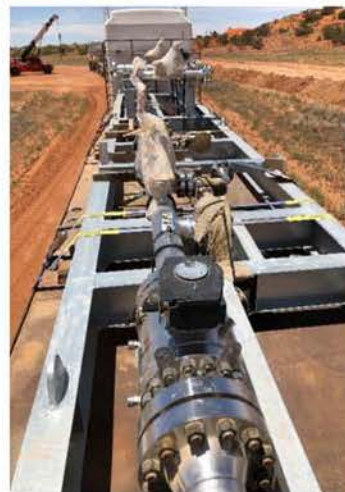
Delivery of manifold skids to Vali site
