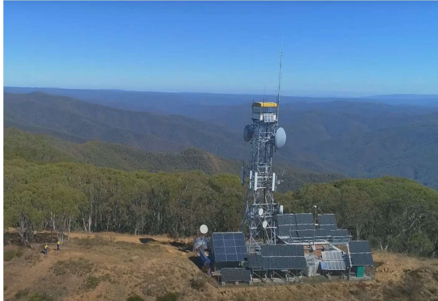
Figure 6. Telstra tower at Mt Terrible, Victoria – powered by solar panels, batteries and permanent onsite diesel generators.
