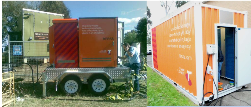
Different Mobile Exchange on Wheels (MEOW) units
